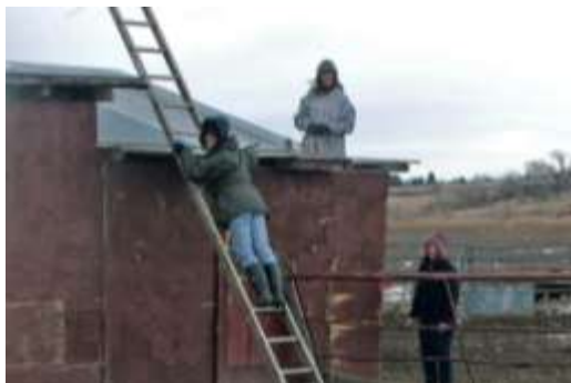
Marie Hackett, Toni Rautus, and Elisa Bilby repair a roof destroyed by 102 MPH winds
