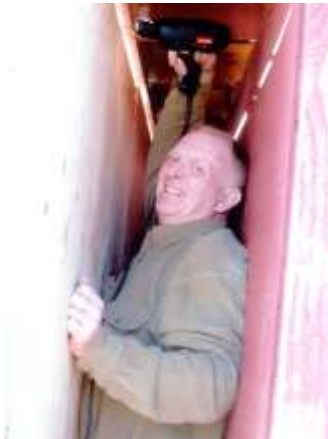
Terry Michel squeezes into tight quarters while repairing a barn at the rescue
