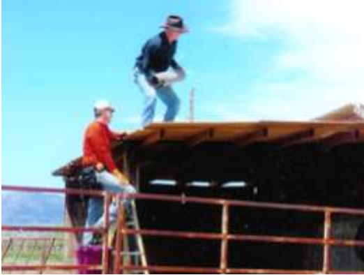
Rob Nixon and Terry Michel rebuild a roof on a wind damaged shed
