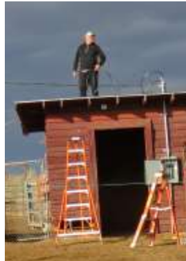
Jeff Marshall works on our electrical in PREPARATION FOR "TANK HEATER" SEASON
