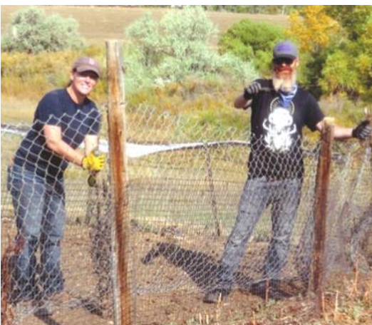
EMILY KIL AND RYAN SHIELDS TAG TEAM A SECTION OF UNRULY FENCE IN ONE OF OUR OLDER PENS
